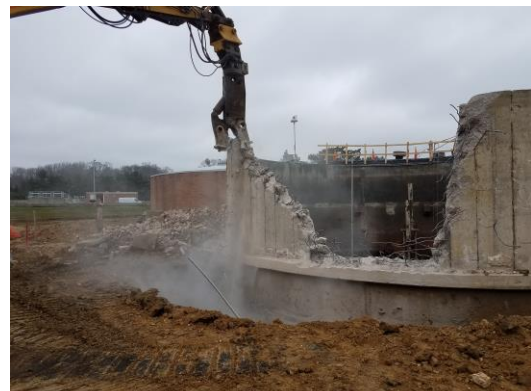
Secondary Anaerobic Digester Demo
