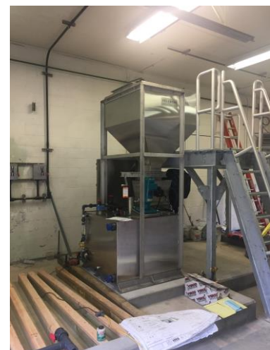
Hydrated Lime Mix System
